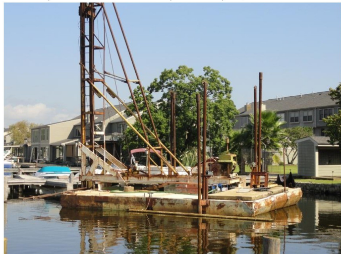
Dewitt Deweese’s pile-driving barge drives new piles to replace the rotted ones. Another two dozen piles await replacement. Old piles will be broken off below grade to insure a safe docking area.
