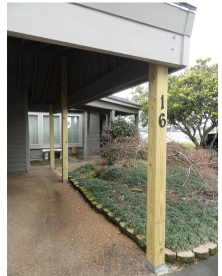
The new posts are elevated on plinth blocks allowing water to run under them
